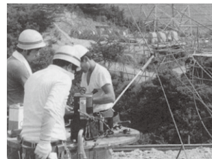
500 kV Seibu trunk line was constructed (completed in 1972)
