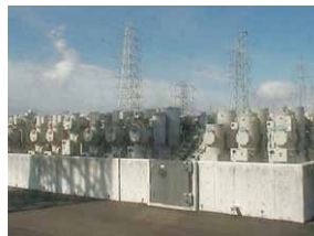
Tsunami protection measures of substation facilities (floodwall equipment)
