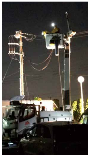
Emergency power transmission by power generation vehicles
