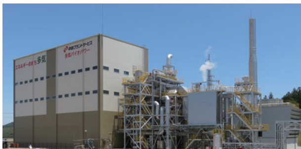
Taki Biopower Power generation scale: 6,750 kW Fuel used: wood chips (ordinary and unused materials)
