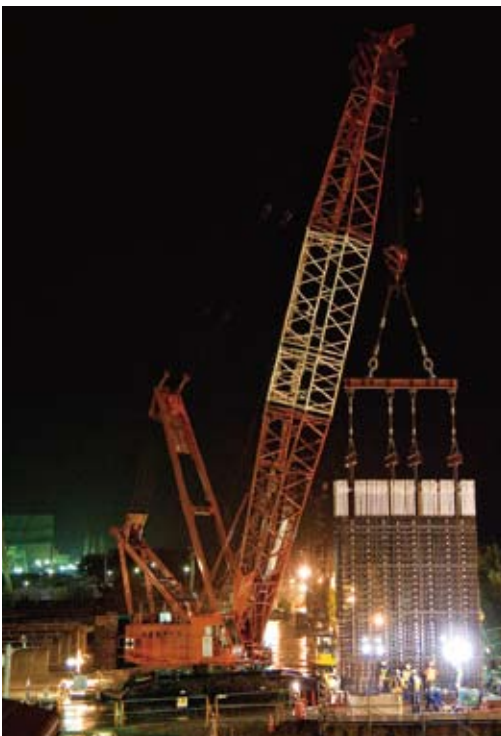
The bedrock was strengthened by the use of 10 m to 30 m long reinforced concrete bases.
