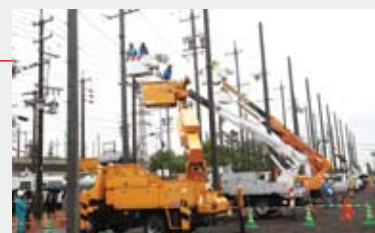
Training on distribution facilities held with the participation of all 10 electric power companies in Japan (Nisshin City, Aichi Prefecture)
