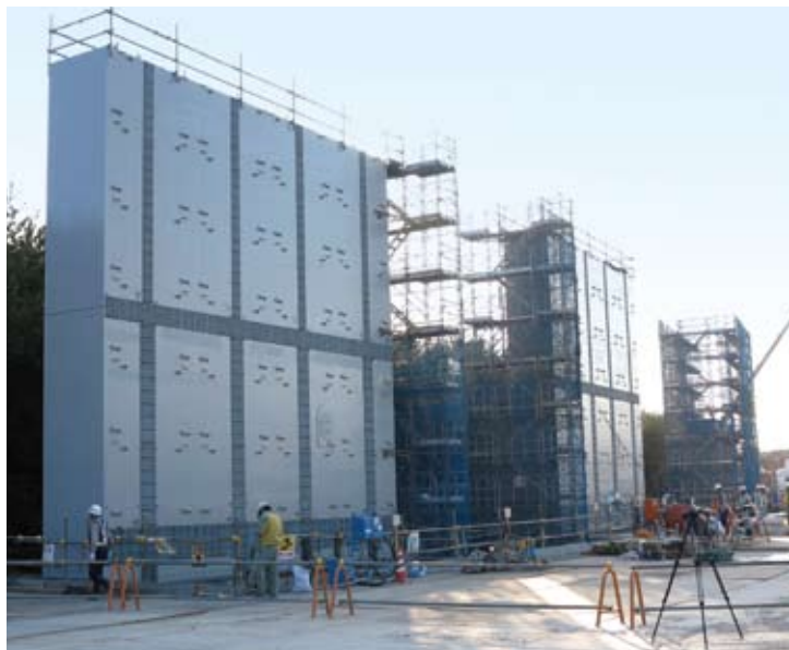
The floor panels and wall panels are being installed one at a time. The panels have metal parts on the surface that are used for the attachment of additional rust-resistant panels.
