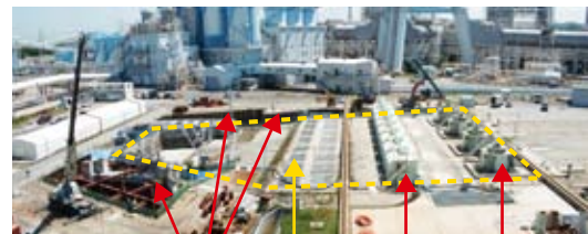
(Seawater on the left side of the photo) Ground reinforcement with the use of concrete and other materials The intake tank is located underground within the area surrounded by a yellow dotted line.
