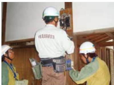
Checking wiring at Mandara Temple in Konan City, Aichi Prefecture, conducted jointly with the Chubu Electrical Safety Services Foundation
