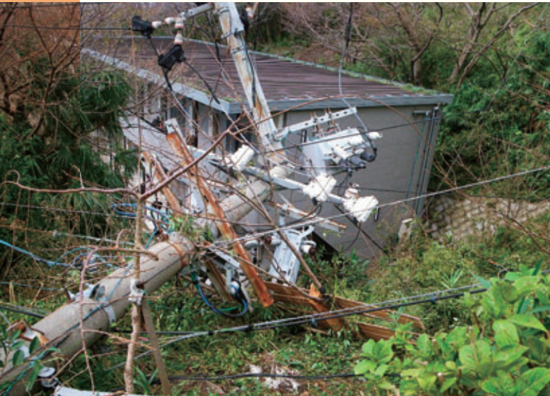
Utility poles damaged by typhoon (Gamagori City, Aichi Prefecture)
