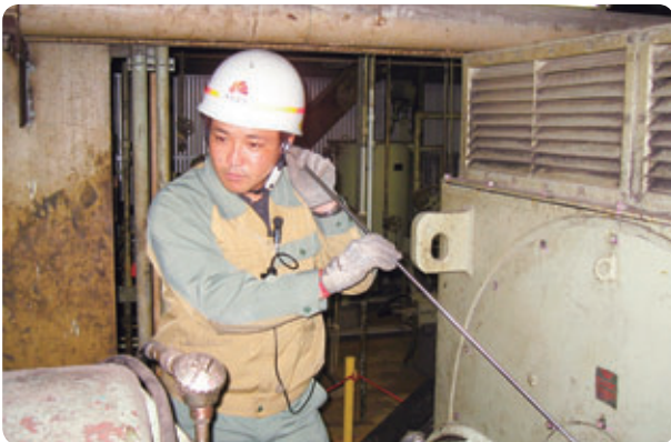
A worker checks the sound of the drive motor in a thermal power plant water supply pump
