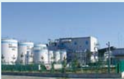
Insulation oil treatment facility
