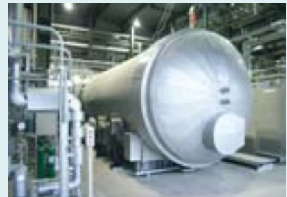
MCFC Cogeneration System
