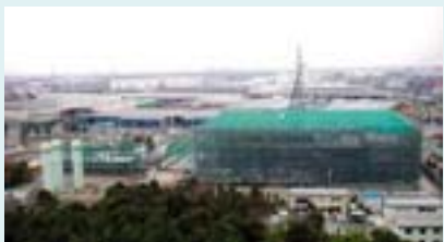
Transformers treatment facility (tentative name)
