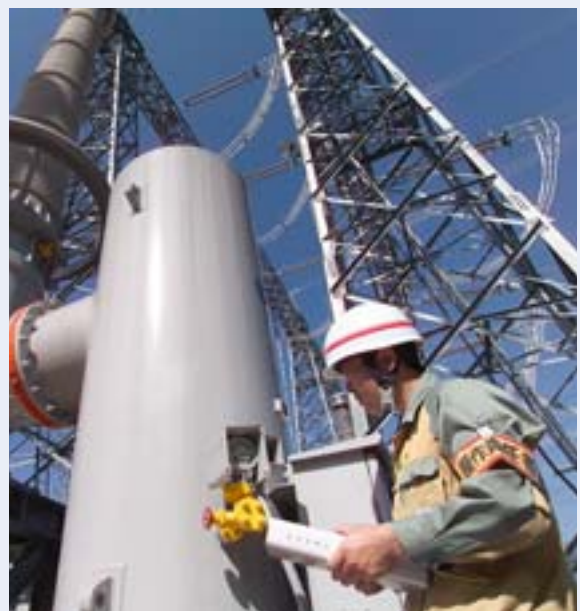
We ensure proper operation of power facilities through periodic checks
